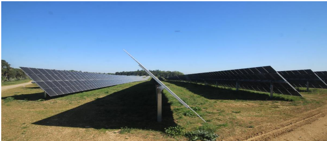
Plate 2-1 Typical Tracker Solar PV Panels in an Angled Orientation
