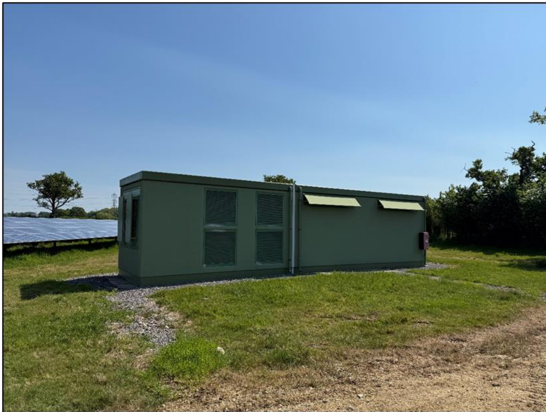
Plate 2-8 Typical 33kV Switch room
