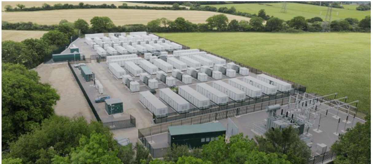
Plate 2-9 Typical Battery Energy Storage System
