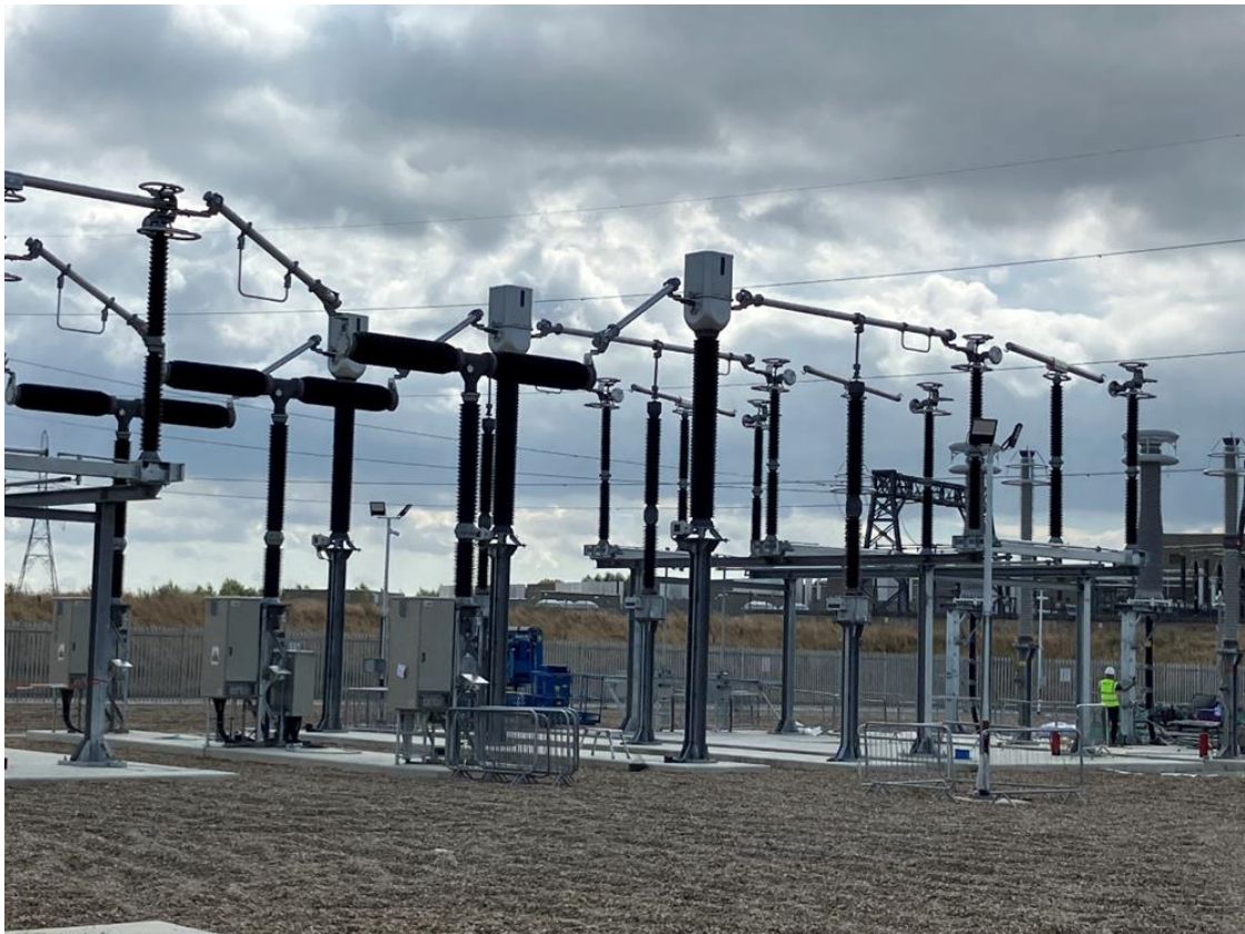
Plate 2-10 Example of equipment at a typical 275 kV on-site substation.
